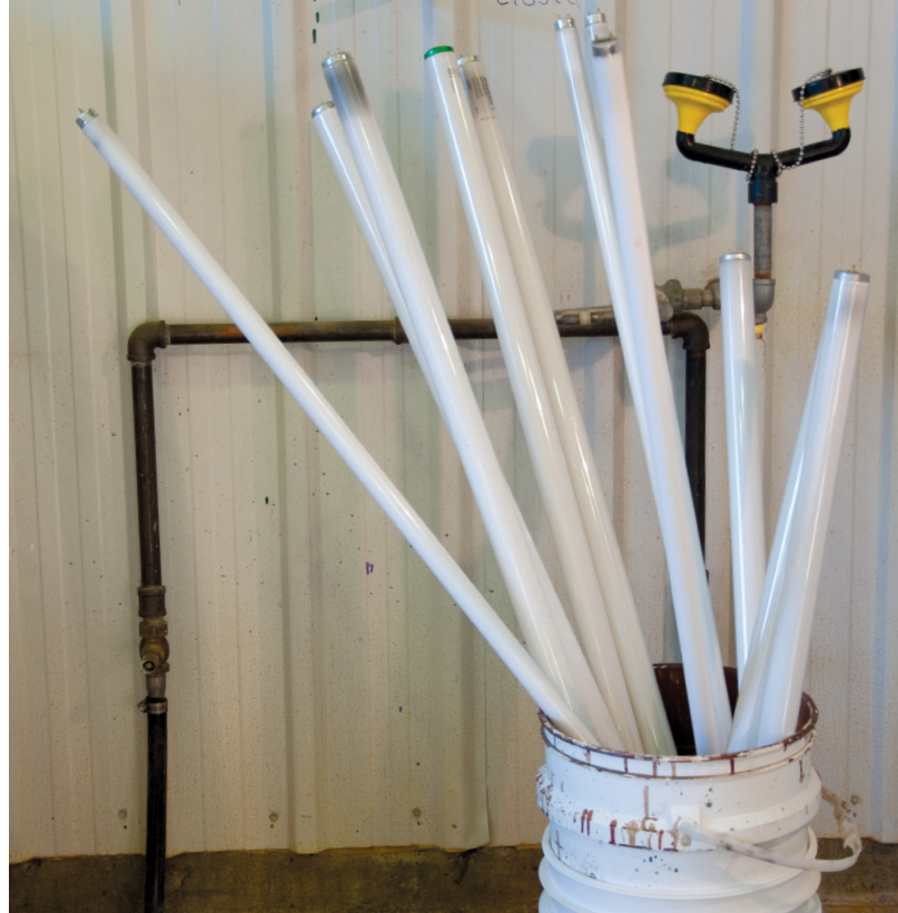
Improper Storage (above) and Good Storage (below)
